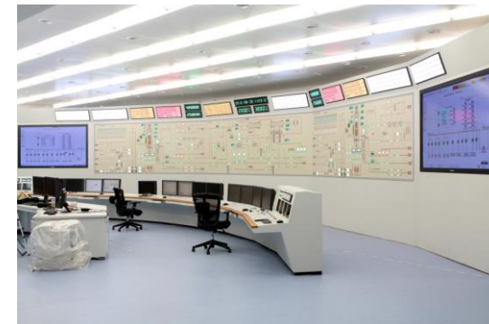
Main control room
