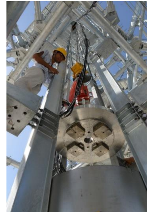
Spent fuel storage system
