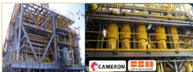
Figure 12. CO 2 compression topside module on FPSO at the Lula field – Heaviest module aboard
