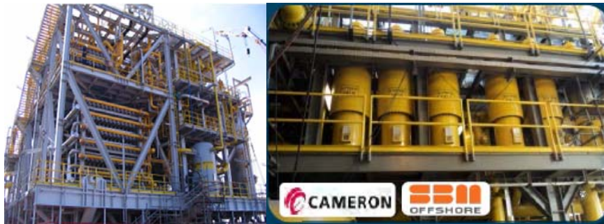
Figure 12: CO 2 compression topside module on FPSO at the Lula field – Heaviest module aboard
