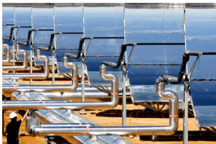
A solar power plant in Alvarado. REUTERS
